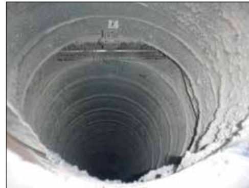
Fire damper installed within a dirty extract duct. Fine dust within the duct poses a fire risk and could hinder the damper from working.
