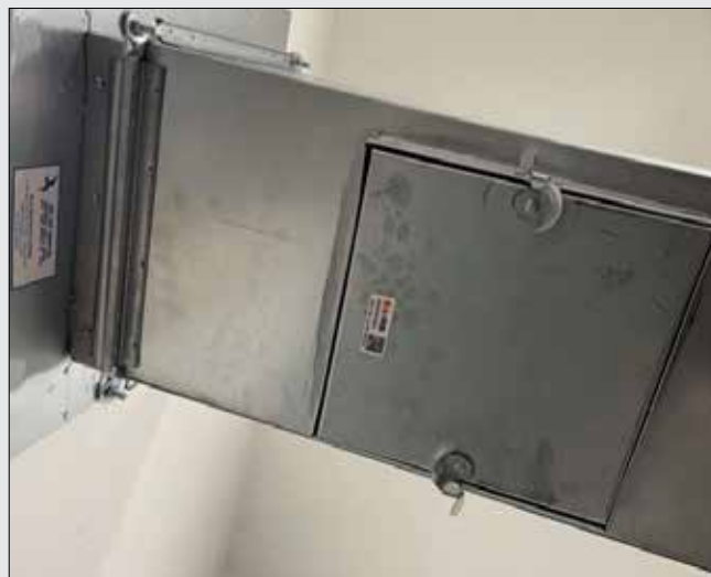
The existing fire damper has a suitable access door and barcode.
