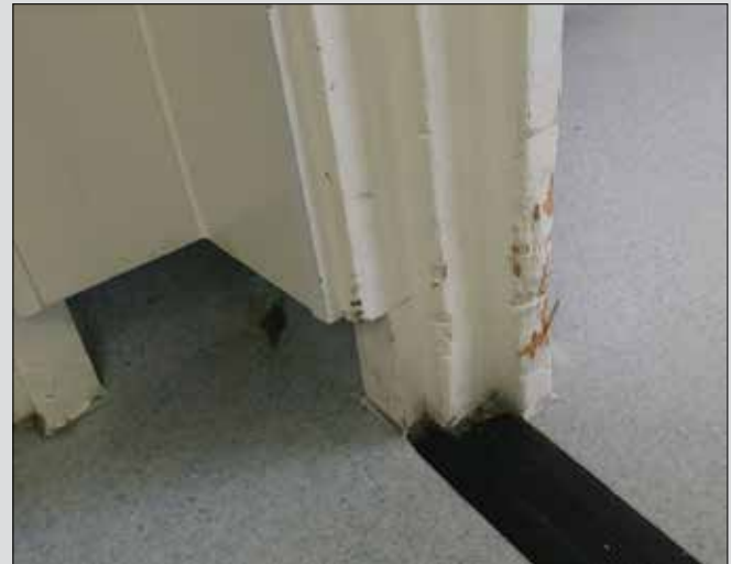
A non-compliant door frame due to repeated impact damage.
