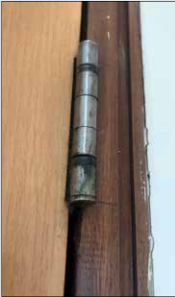
A hinge which has sediment buildup and grime due to lack of maintenance.
