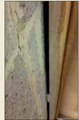
The gap between the frame and wall has been left unsealed.
