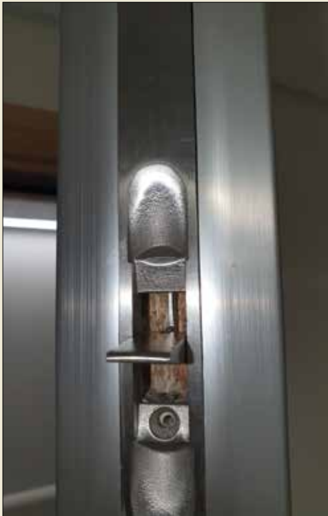
An example of missing intumescent protection to essential ironmongery.
