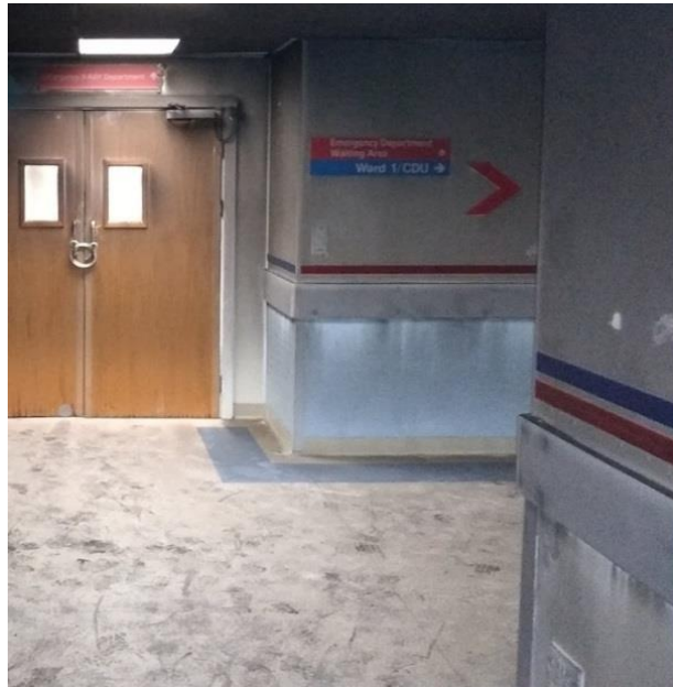
Photo 9 - wall glamour / artwork on the ED corridor - melted but not significant in terms of fire spread
