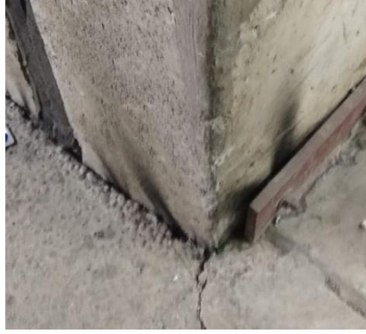
Photo 9 - plant room immediately above the fire showing slight smoke staining
